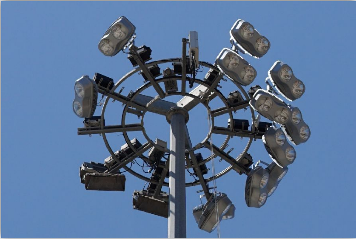
View of a ring with 400WP at 42m height. Noatum. Valencia. Spain
