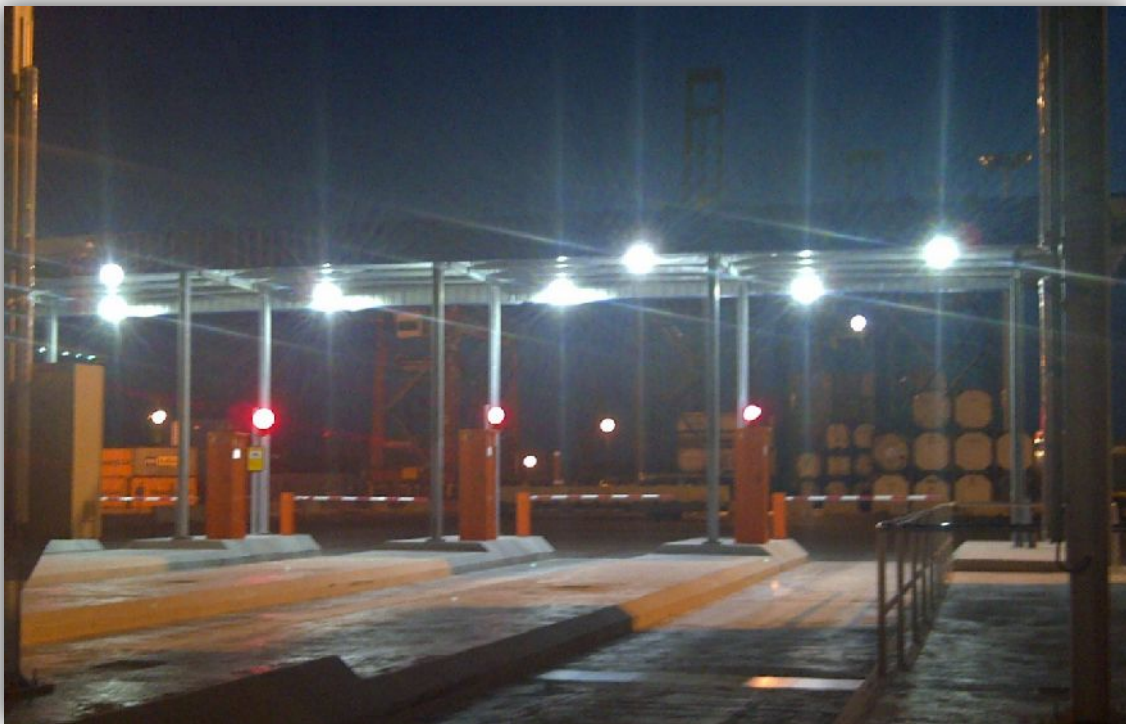
At other side, the view of another gate with 65% less of energy consumption.
