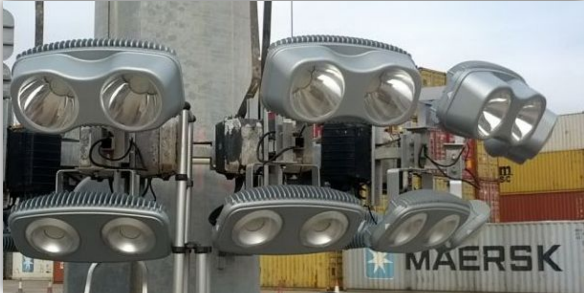
Detail of mounting to have a good lighting performance at Noatum Port Terminal, Valencia, Spain
