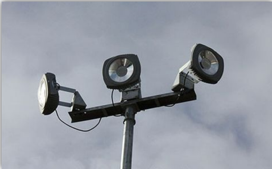
View of three 120° Zihai Luminaire in a Pole.
