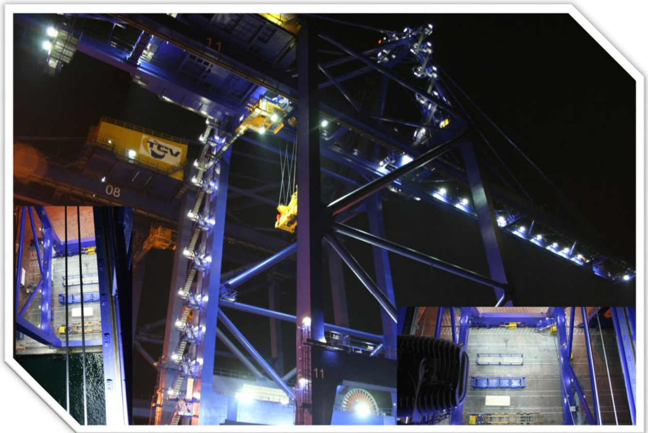
First Full LED STS Crane installed in TCV at Valencia (by EDAE)
